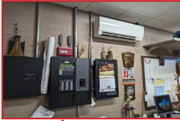
Fire Alarm Panel
