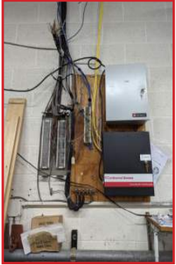
Access Control System
