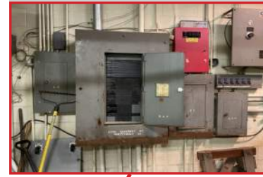
Original Electrical Panels
