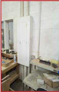
Older Electrical Panel
