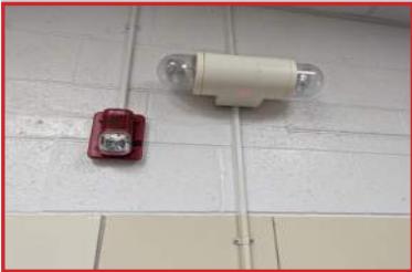
Fire Alarm Horn / Strobe and Egress Light
