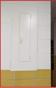
Older Electrical Panel
